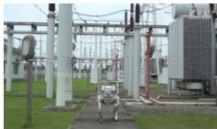
Jinan Substation Intelligent inspection
